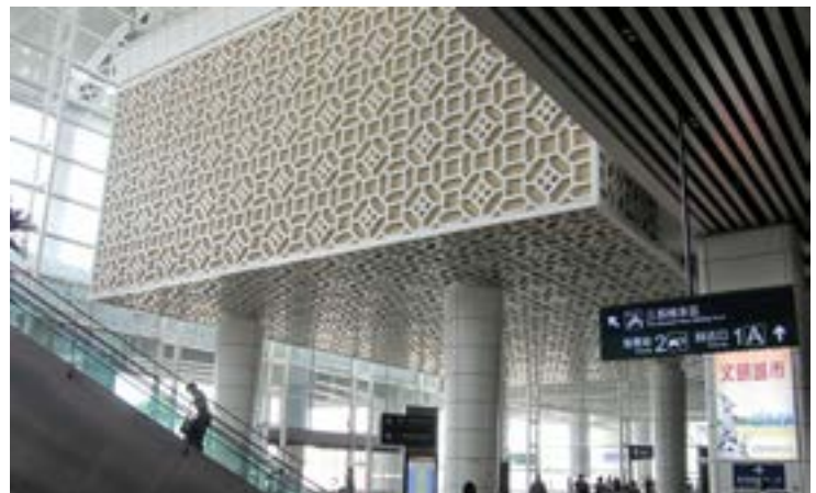
South Guangzhou Railway Station: Class A fire-rated vermiculite panel attached on the ceiling for both decoration and fireproof features.
